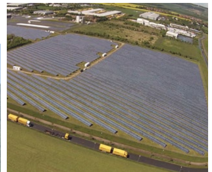
Ground-mounted System 6.092,24 kWp Nohra, Germany
