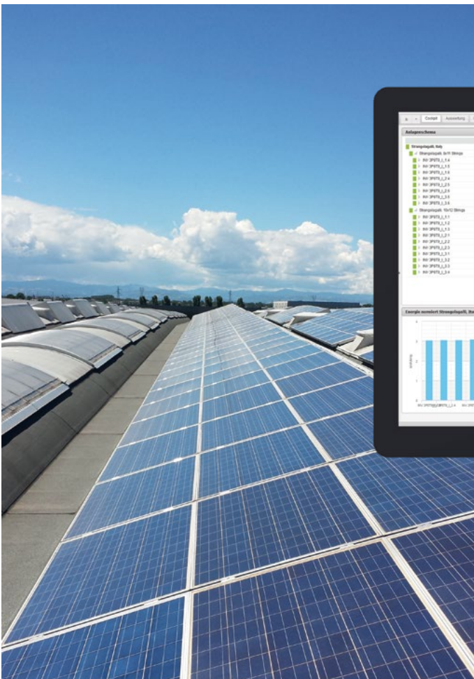
Rooftop Integrated System 1.376,32 kWp Monticelli, Italy
